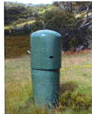
Figure 4: Photo of a hydrant.
